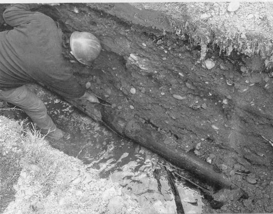
REPAIR CONCERN: An Aqua America worker tends to broken pipes. Some argue that private companies can build and repair water distribution systems cheaper than governments.
